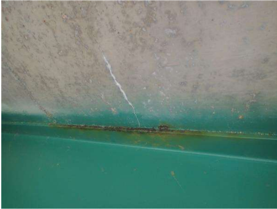
Photo Number: 5 Photo Taken: 02/28/2023 TRANSVERSE CRACKING WITH EFFLORESCENCE AND CORROSION AT BEAM TOP FLANGE
