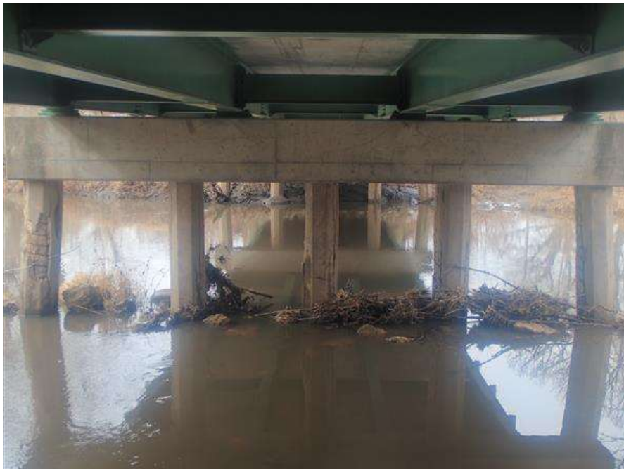
Photo Number: 6 Photo Taken: 02/28/2023 CRACKING, DELAMINATED, SPALLING WITH EXPOSED CIRCUMFERENTIAL REINFORCING AT EAST PIER PILE ENCASEMENTS
